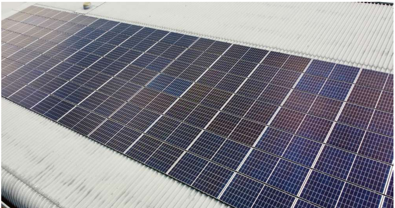
MACALPINE Road Fire Station Solar PV
