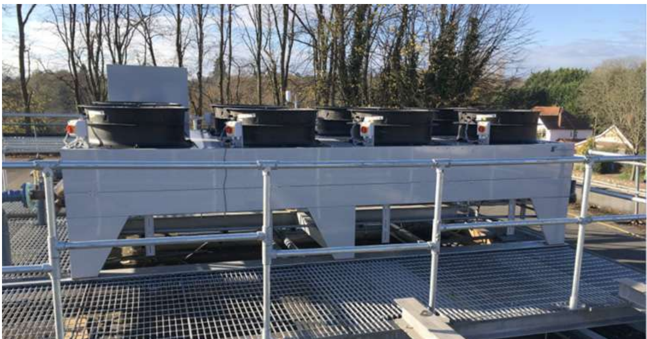
Figure 2 – Roof mounted dry-air coolers
