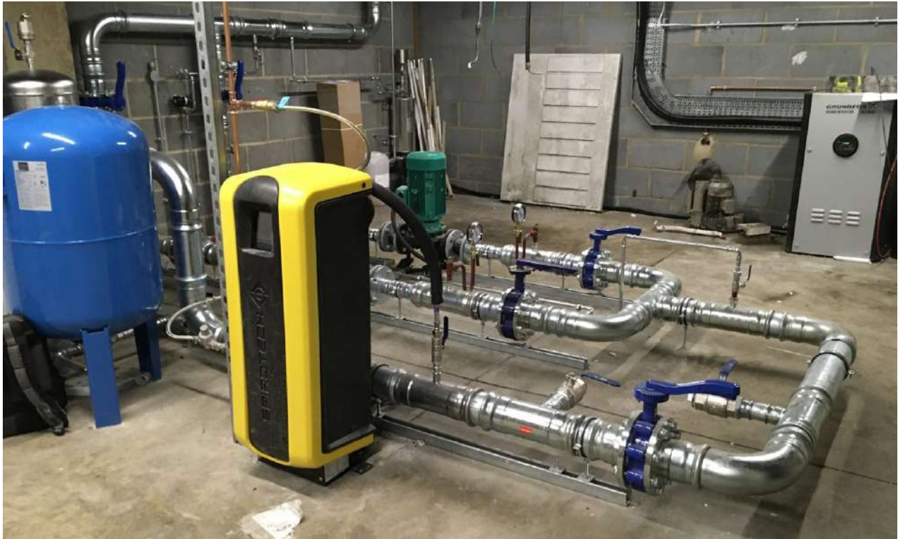
Figure 3 – Internal pump station for the water chilled loop
